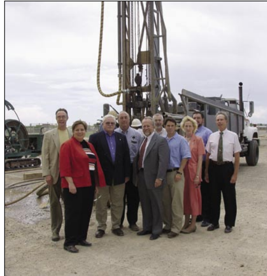
Dedication of phase one of Alamogordo High School's new geothermal heating and cooling system. Water conduits being installed.
