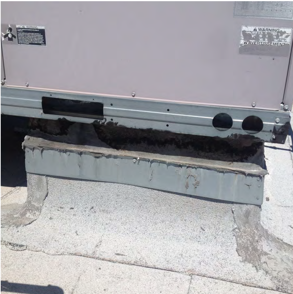
Example of HVAC unit (curb perpendicular to positive roof slope)
