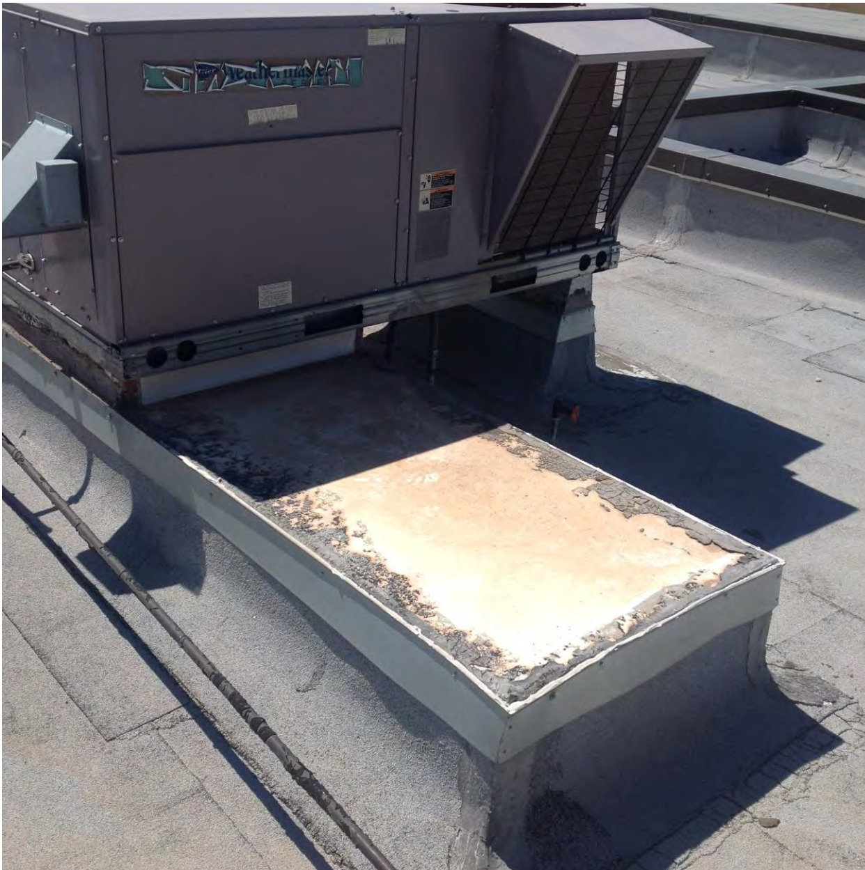
Example of old re-used (oversized) curb to accomodate replacement HVAC unit. Water accumulates at top w/ no positive drainage.
