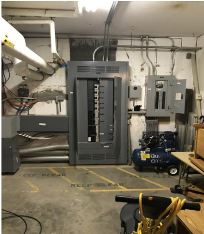
Panel "P" located in basement of building 200.
