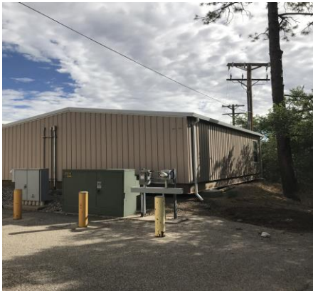
LACUD 300kVA transformer-2311
